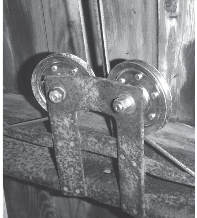
Figure 1: Emergency Brake Cable Pulleys
